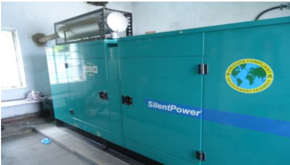
Photo of Generator which will shift from existing location to Near DGPS station of IWT Terminal.
